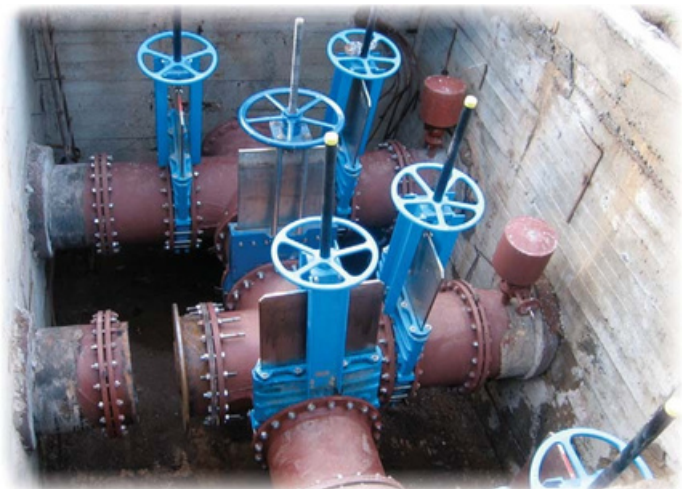
Sewage water treatment application
